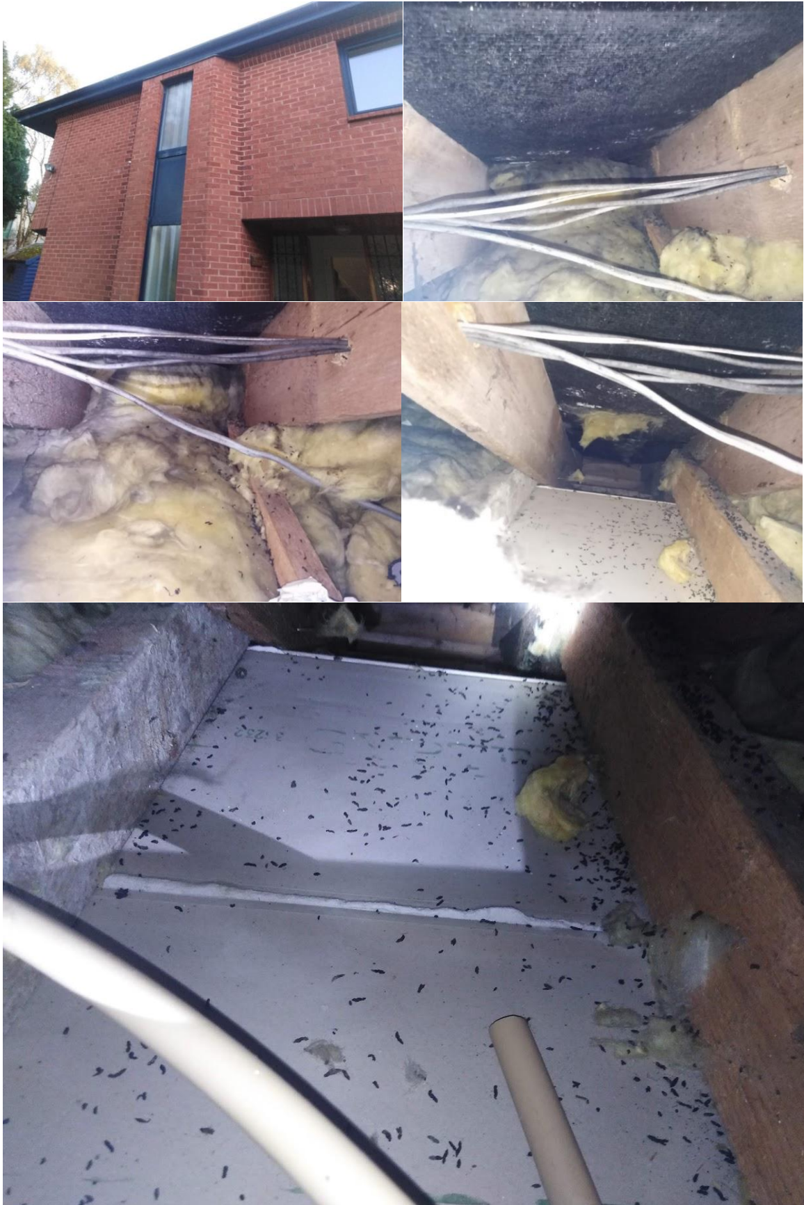
Plate 4: Bat roost evidence in 97A Highfield Park
